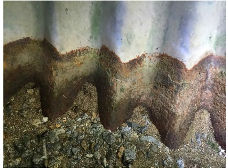
Pitting & Flaking of Culvert Floor
